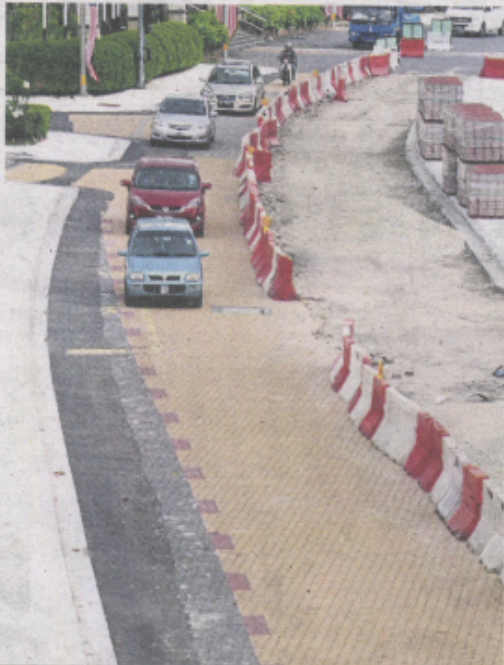
(Above) Business operators are complaining about the dust caused by the project in Jalan Yong Shook Lin.
